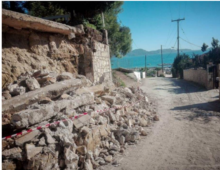
Picture 10. Collapse of a stone retaining wall following Zakynthos earthquake (Source: https://www.cnn.gr )
