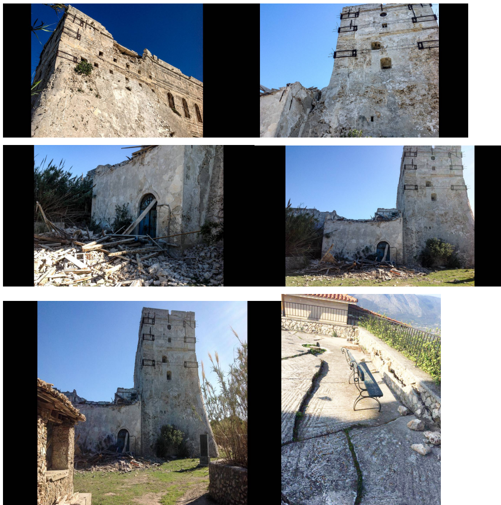
Picture 14. Observed damage at the Castle-Monastery at Strofathes island
