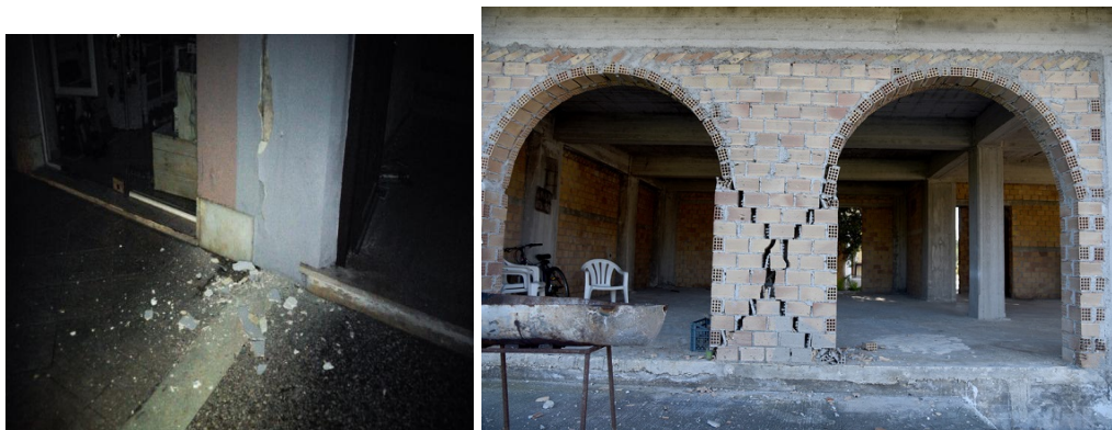
Picture 13. Observed damage at Zakynthos town
