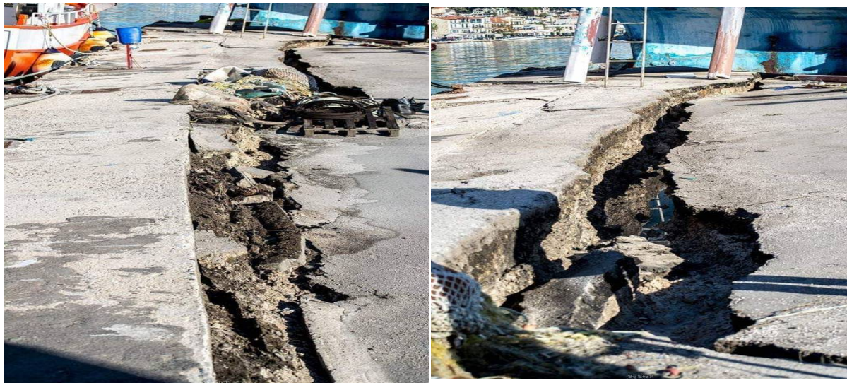
Picture 2. Lateral displacement and tilting of the quay walls at the port of Zakynthos
